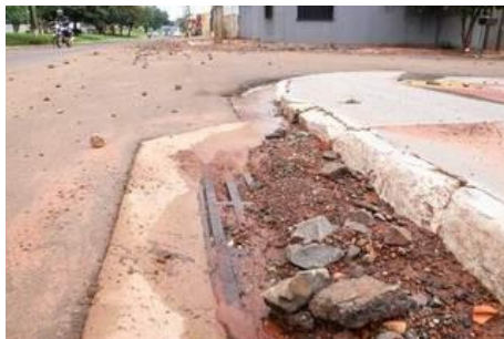
Fig. 9 Obstruction of storm drain at Segredo UHM
